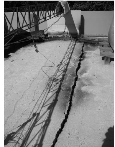
Fig. 6 Crack above intermediate beam first test
