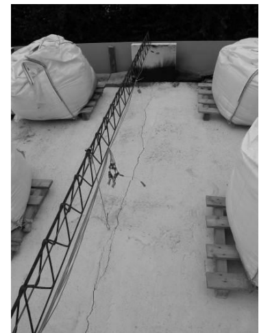
Fig. 8 Crack above intermediate beam second test
